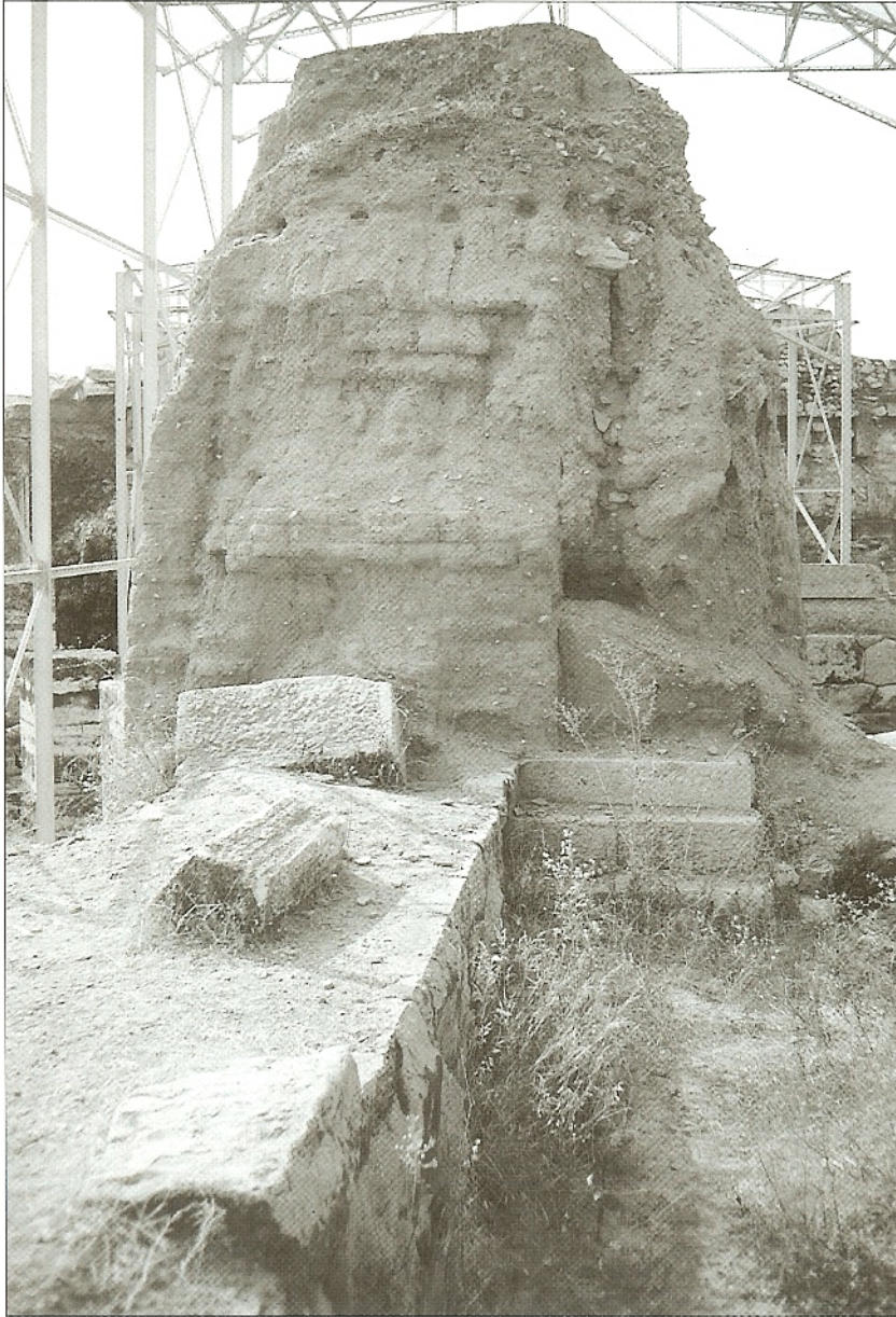
At Eleusis the tyrant Peisistratos (d. 527 BC) enclosed the sanctuary of Demeter with a substantial circuit. This was built with a low socle of limestone blocks set in polygonal style, which carried several metres of sun-dried mud-brick. (Author's collection)
